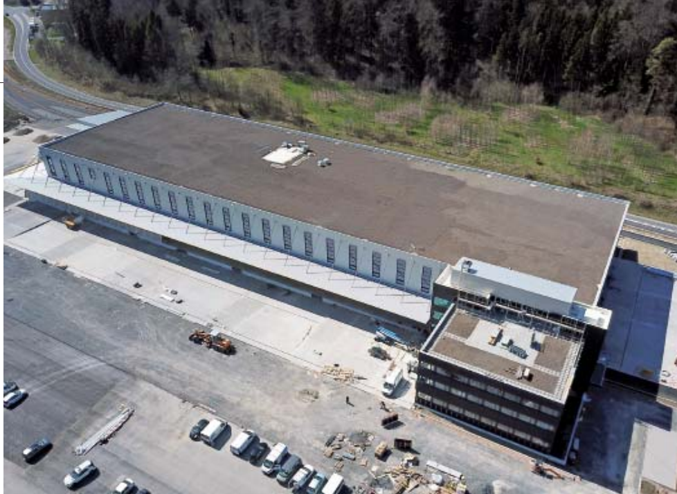
CT worked under a provisional emergency roof to finish the new logistics centre on time.
